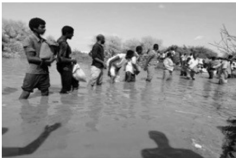
Figure 5. A human chain is created to transport sandbags to the site selected for the new dam. Source: RUS Team
